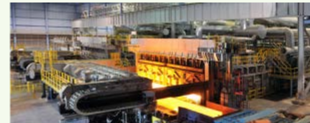
Walking Beam Furnace 300 tph
