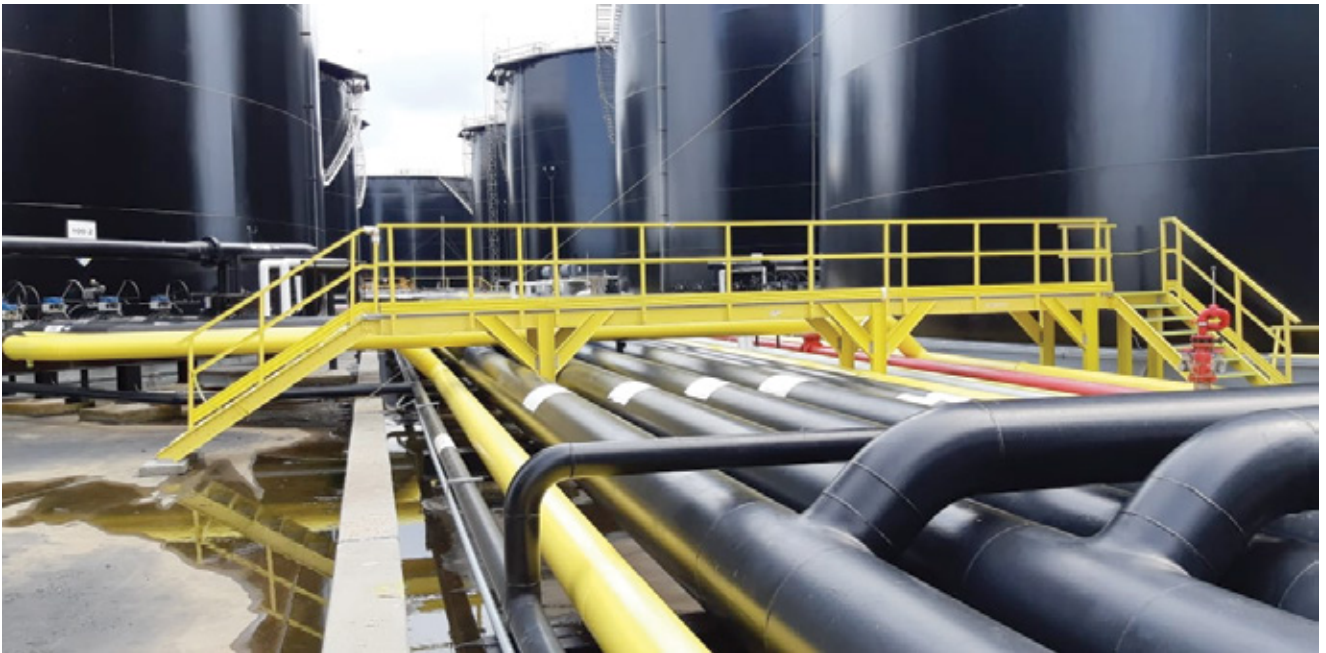
FRP crossing of the tank containing pipelines
