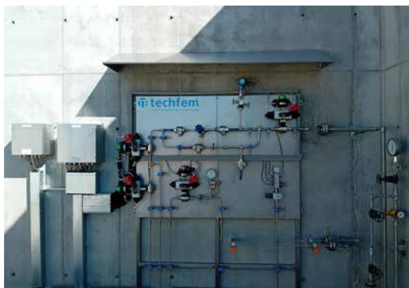
Control and safety panel of the Hyround plant in Sestu
