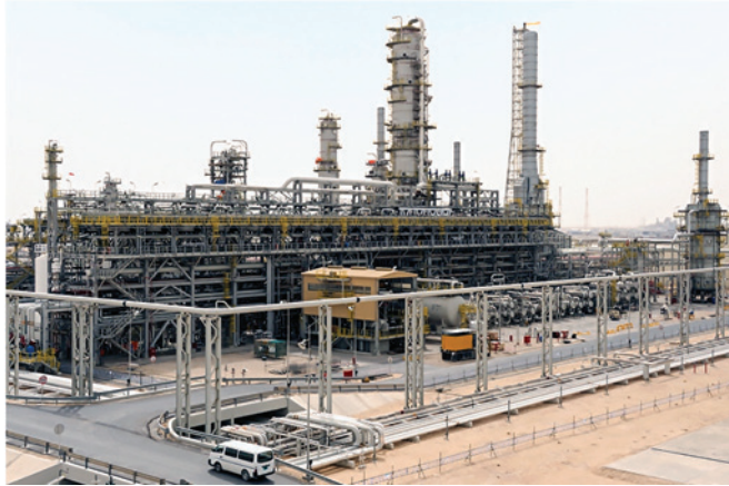
Fig. 4 – A Qatar Petroleum-led JV is constructing Laffan Refinery 2 (LR2), a $ 1.5 B refinery that will process untreated condensate produced from Qatar's North field
