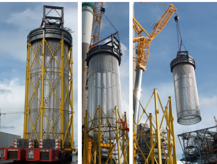
Fig. 7 - One modularized coil hanged on top part (arch), lifted from its frame structure to final destination
