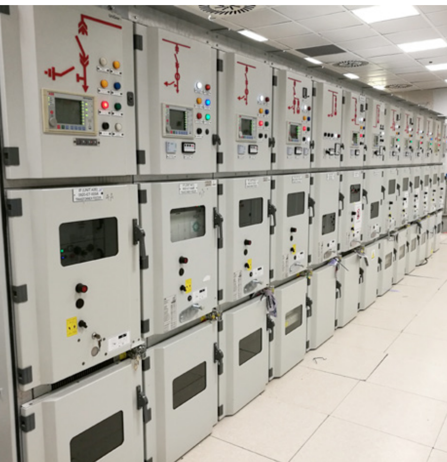
Fig. 3 – The Medium Voltage Switchgear
