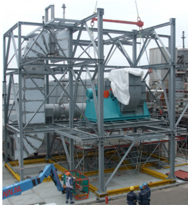
Fig. 5 - The biggest module (still uncompleted) during site prefabrication in the pre-turnaround phase
