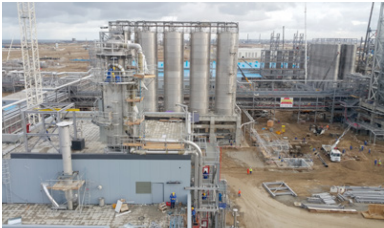
Detail of the PP unit – dry end
