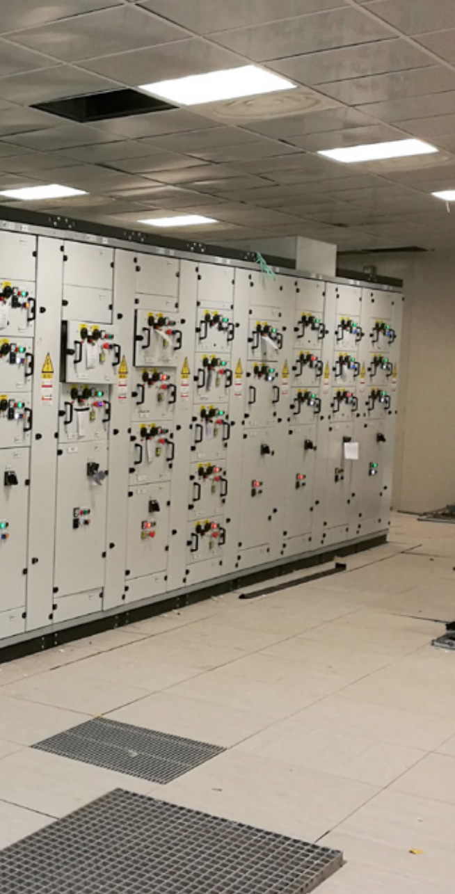
Fig. 1 – The Power Motor Control Center
