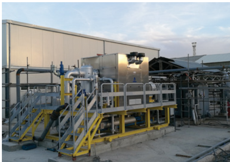
Another successful installation - Unit: IA package with oil-free compressor 3200 Nm 3 /h; Location: Jordan onshore refinery Zone 2
