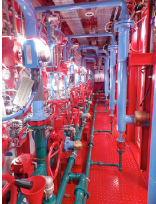
Deluge valve: typical container, interior layout
