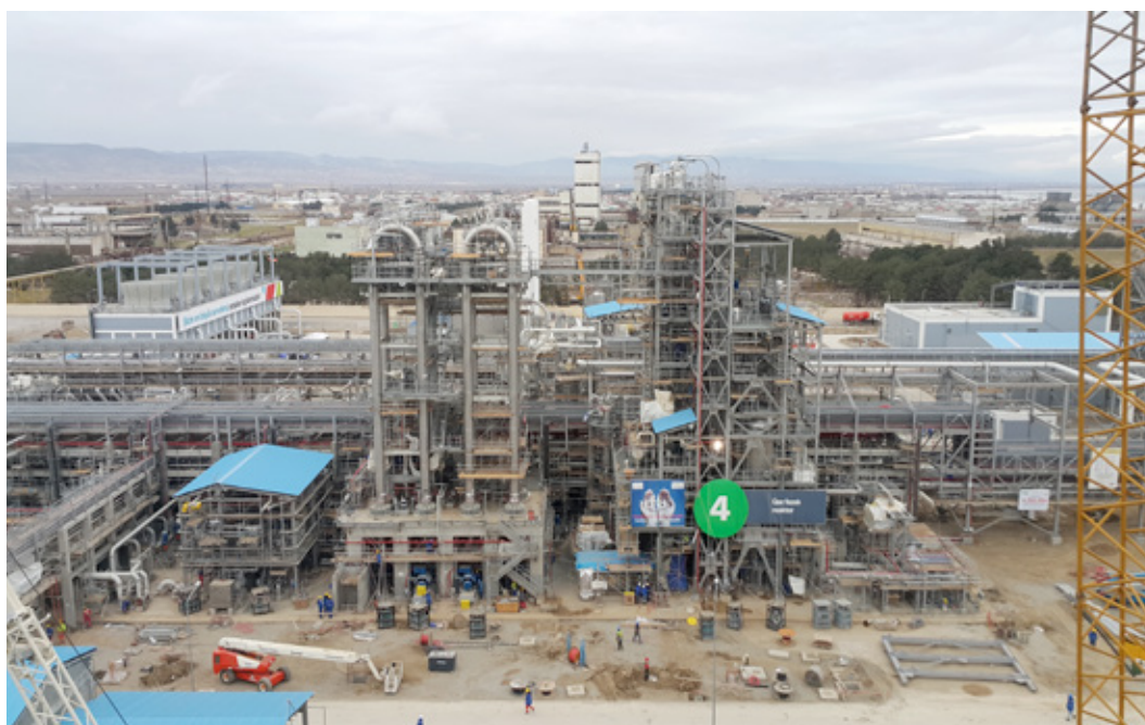
Detail of the PP unit - wet
