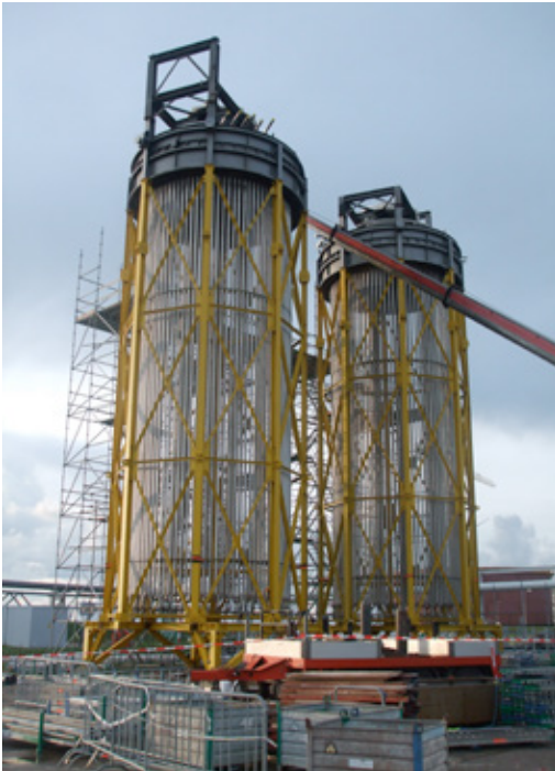
Fig. 4 - Modularized radiant coils hanged on top part (arch) inside their temporary frame structures
