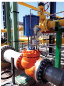
High Performance 12" Globe Valve, Oil & Gas Plant, Argentina
