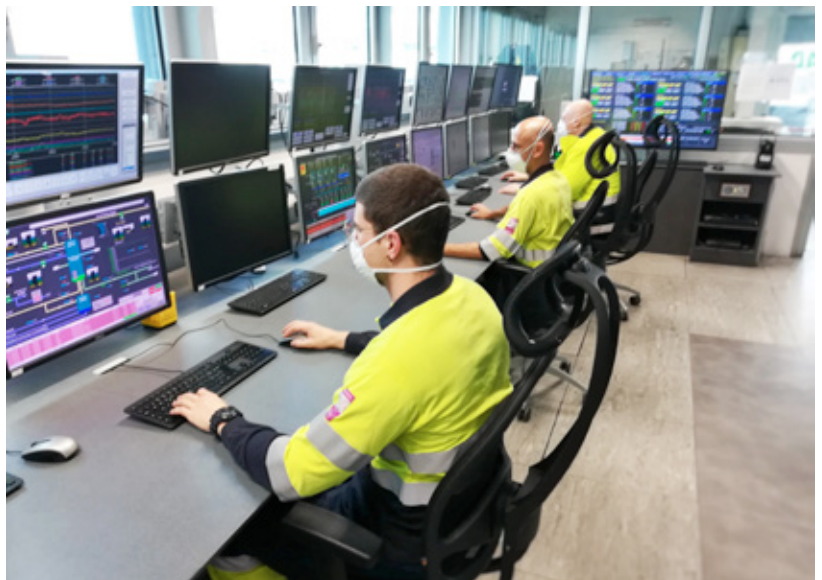
Picture 6: SIAD MI control centre
