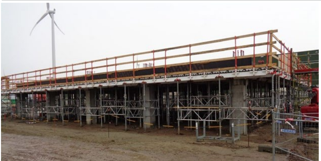
Figure 59 Example execution of an integration of precast approach and cast in situ activities (2/2)
