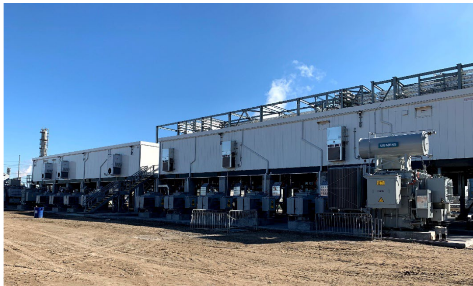
Figure 42 Example of modularized substations
