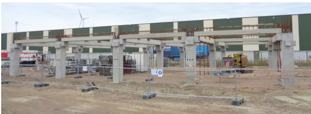
Figure 58 Example execution of an integration of precast approach and cast in situ activities (1/2)
